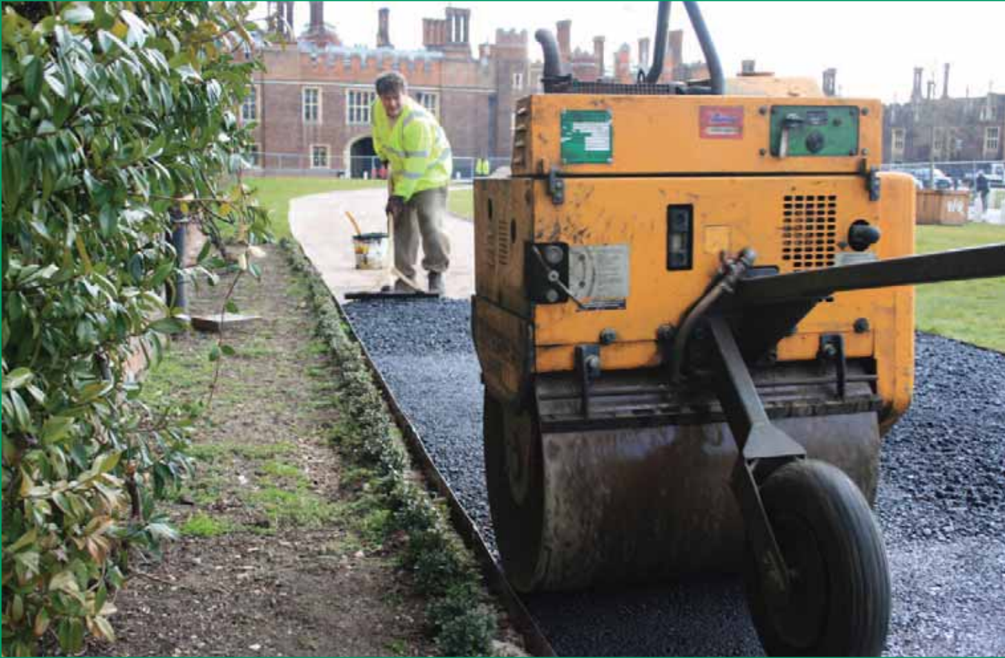
Walkways were excavated between the long Barrack Block building and the main palace building.
