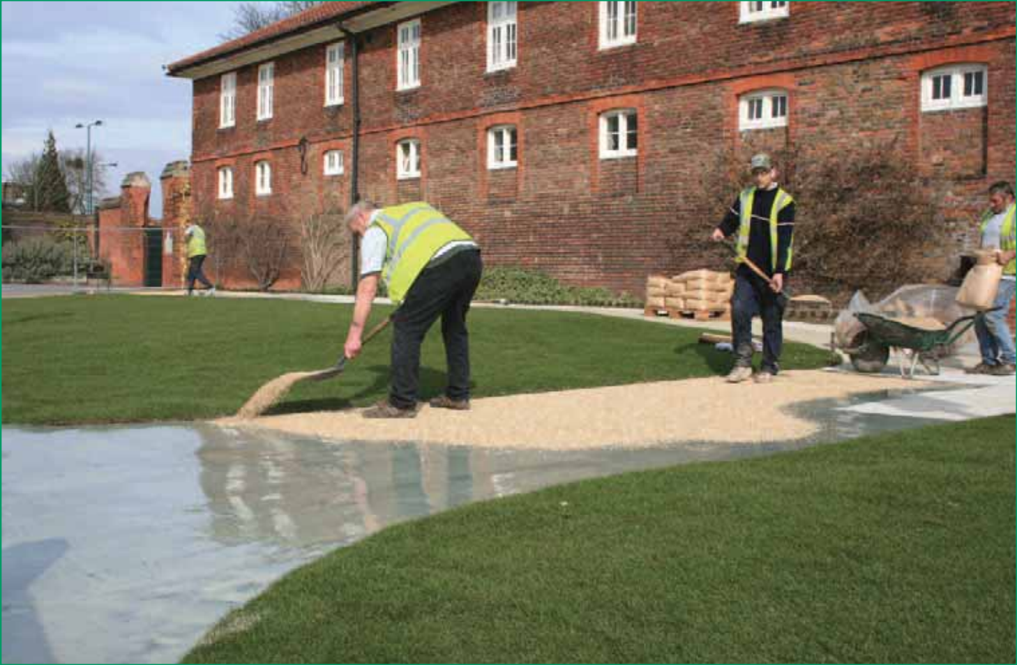
Gravel was spread onto the resin-bonded surfaces giving a durable and attractive walkway.
