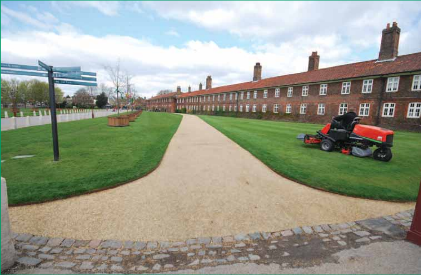
The finished walkways with new turf laid and tied into existing banks of turf.
