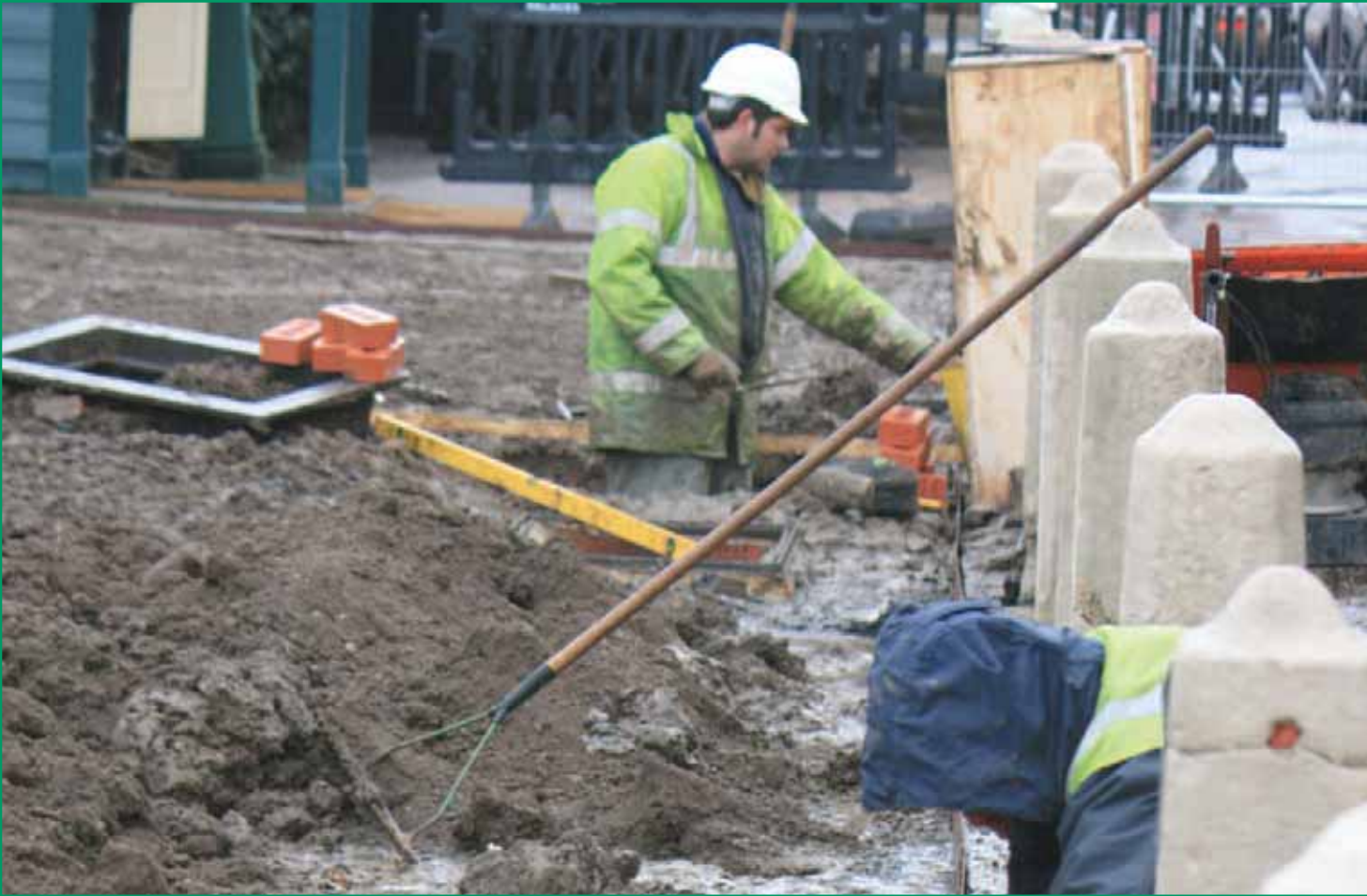
Tarmac was removed from the road edges to a width of 3m, revealing services which required updating.
